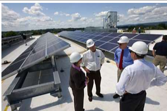
Solar array powering much of the Campus Square building at PERC member HACC.
